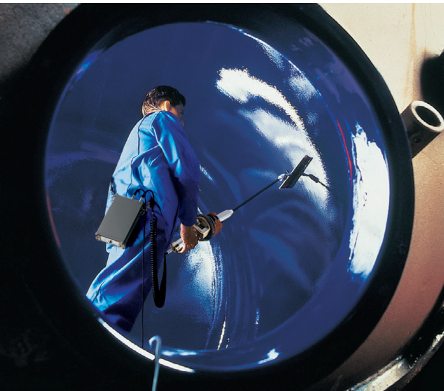
Pore testing of the enamel coating of a boiler, using the POROSCOPE®
